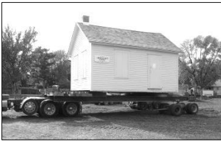
Hoggatt School was hoisted up onto a trailer and placed on a new foundation in December 2013.
