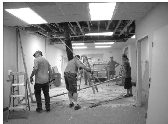
In the former tenant space in suite 100, walls were removed to create open space for exhibits, presentations and a new reception area.
